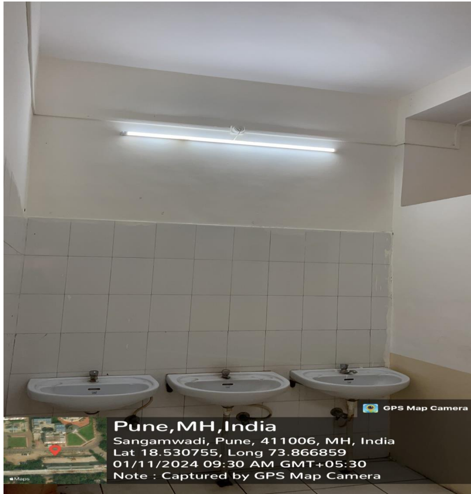
Sensor Based LED Lights (Dimming Type) Installed at Washrooms - AISSMS COP, Pune
