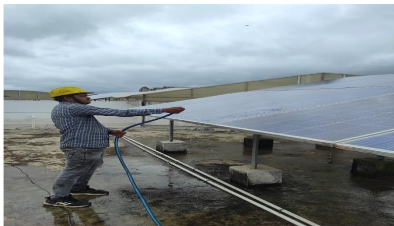
Roof top Solar panels
